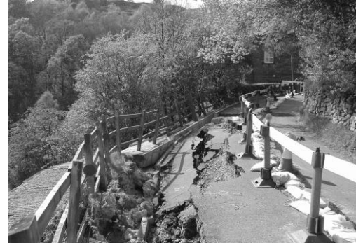
(b) Collapse of road pavement
