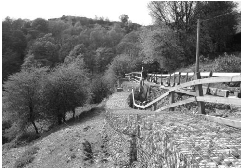
(a) Down-slope movement of existing gabion wall
