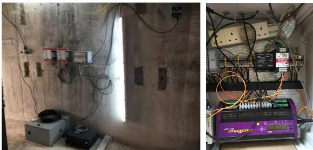
Figure 5.3: Picture of accelerometer and data logger used in full-scale monitoring
