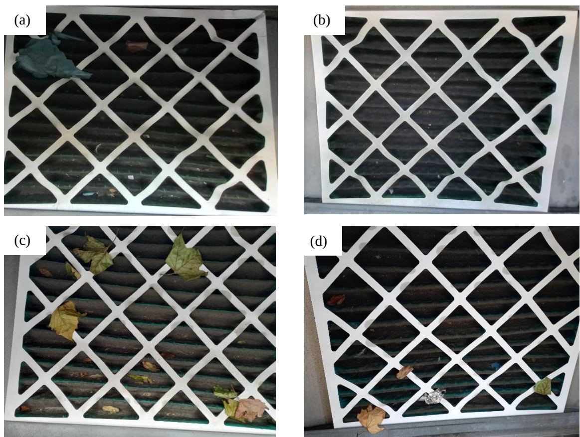
Figure 75. Images of the panel filter condition at end of testing period (a) Control AHU panel filter in AER Case 1 comparsion (b) AER Case 1 panel filter (c) Control AHU panel filter in AER Case 3 comparsion (d) AER Case 3 panel filter.
