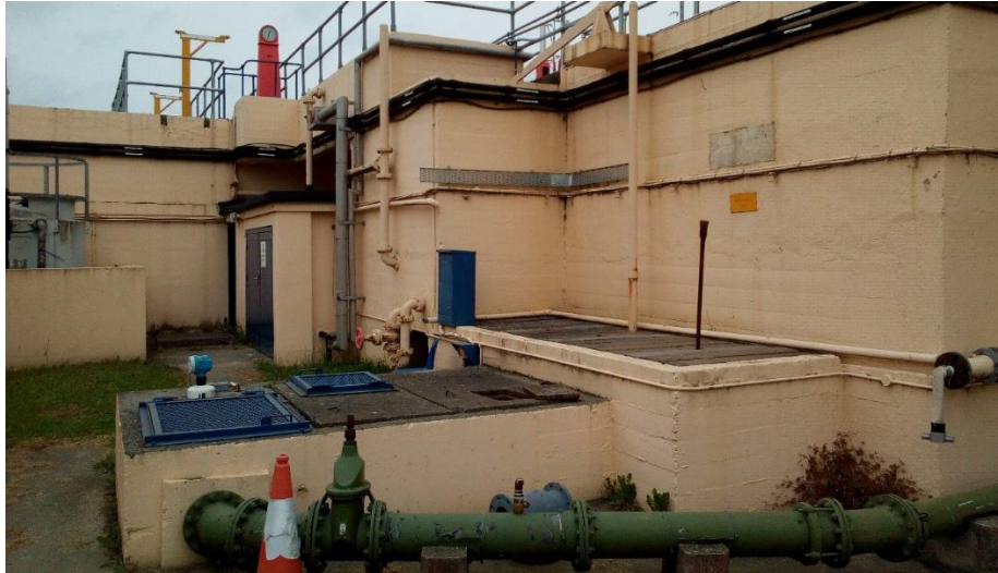
FIGURE 0-26. THE WATER INLET AT BALLYBODEN WTP
