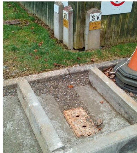
FIGURE 0-28. THE LOCATION OF FLOW CONTROL VALVES AT BOHERNABREENA RESERVOIR CAR PARK AS SEEN ON 13/06/2018
