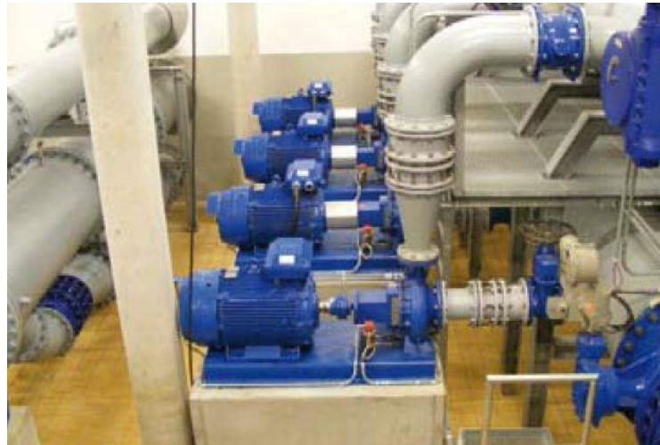
FIGURE 3-37. POWERHOUSE OF BREECH ENERGY RECOVERY STATION (KSB, 2008).
