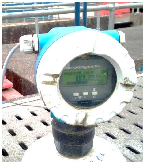
FIGURE 0-27. RAW WATER FLOW METER AT BALLYBODEN WTP AS SEEN ON 13/06/2018
