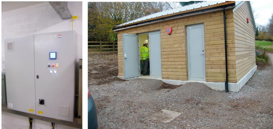
FIGURE 3-38. PICTURES OF THE PAT INSTALLED BY SOUTH WEST WATER ON THE ERME STREAM (KSB, 2013).
