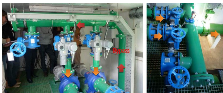
FIGURE 3-36. VIEW OF PAT INSTALLATION AT BELICHE WATER TREATMENT PLANT (RAMOS, ET AL., 2014).
