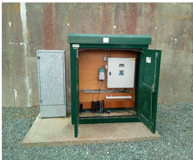
FIGURE 0-41. ELECTRIC CABINET AT RATHNURE TANK WITH VISIBLE FLOW METER AND LEVEL TRANSDUCER AS OF 25/8/2017
