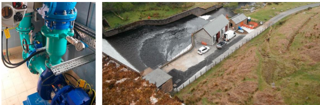
FIGURE 3-34. CENTRIFUGAL PAT INSTALLED AT THE AVON DAM (LEFT) AND VIEW OF THE POWERHOUSE FROM THE DAM CREST (RIGHT) (KSB, 2012A).
