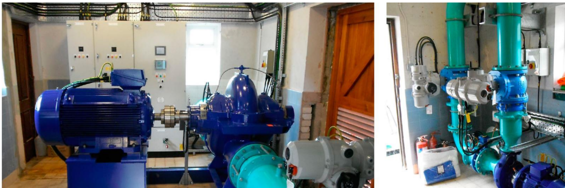
FIGURE 3-33. IMAGES OF THE TWO PATS INSTALLED AT AVON DAM: SPLIT-CASE DOUBLE FLOW UNIT (ON THE LEFT) AND CENTRIFUGAL UNIT (RIGHT) (KSB, 2012A).
