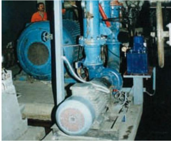
FIGURE 3-41 - PAT INSTALLED IN ŁOMŻA MUNICIPAL HEATING PLANT (EUROPEAN DIRECTORATE FOR TRANSPORT AND ENERGY - FP6 PROJECT SHAPES, 2010).
