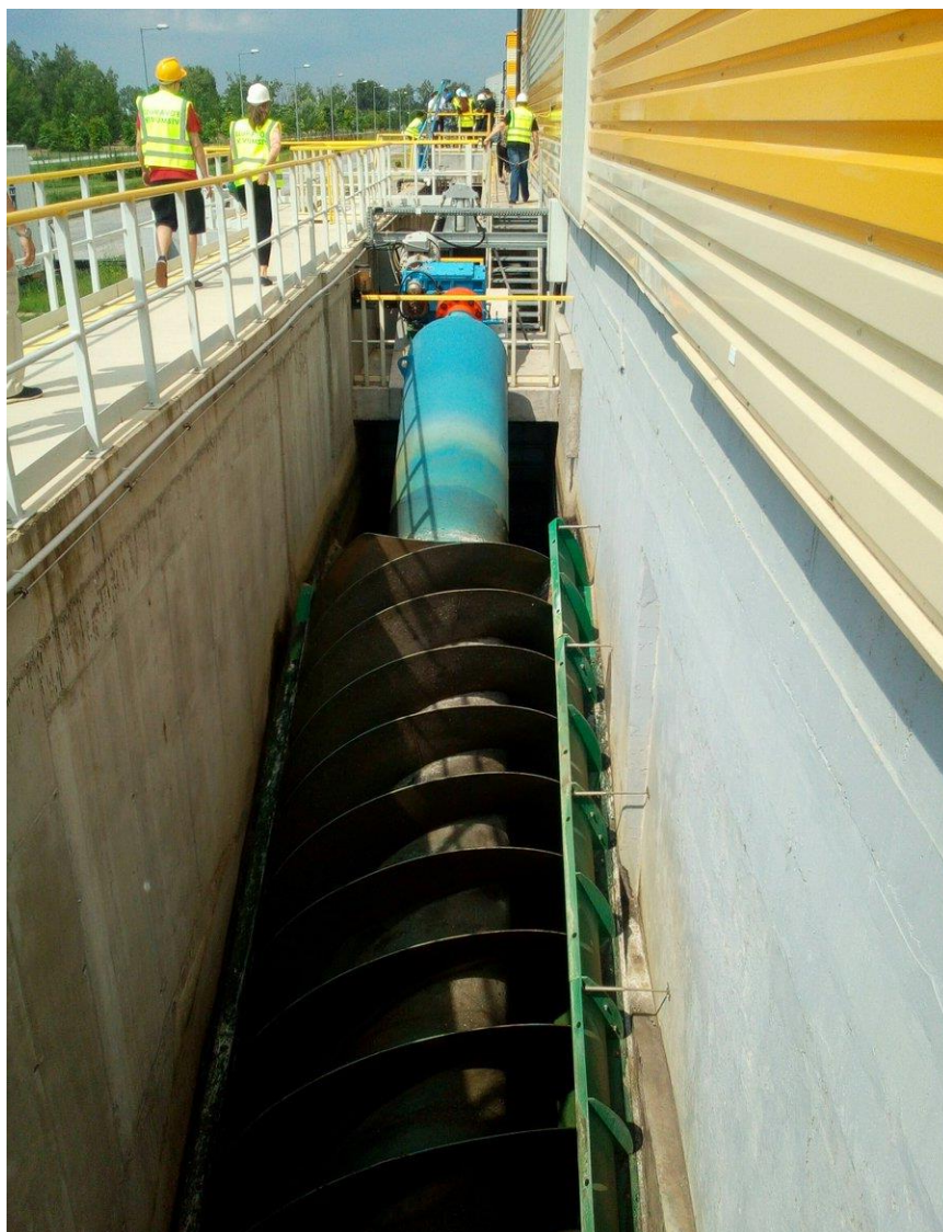
FIGURE 3-12. THE 75KW ARCHIMEDEAN SCREW CONVERTER AT CSEPEL ISLAND WWTP, HUNGARY.
