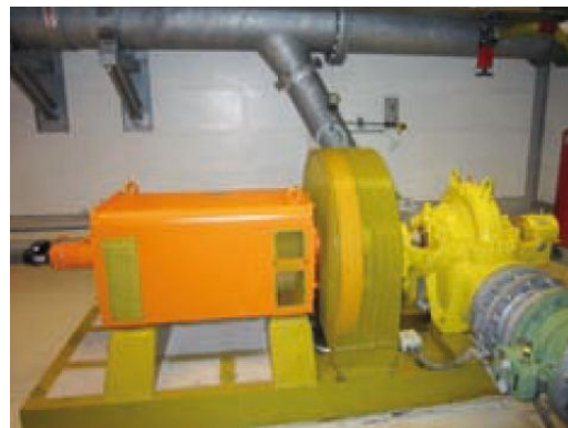
FIGURE 3-35. PAT INSTALLED AT THE OUTFALL OF NYON WWTP.
