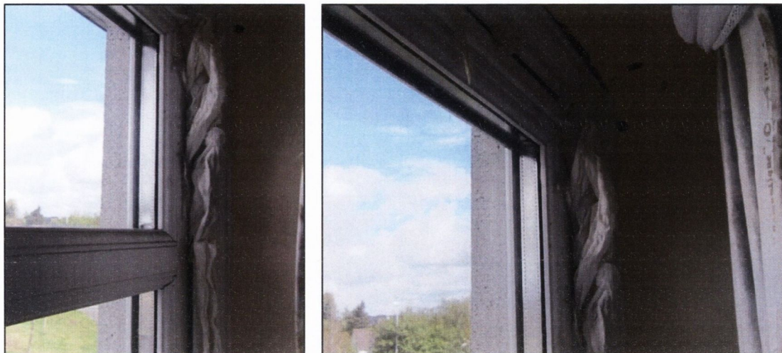
Figure 42 Poor window seal blocked with kitchen paper in Dwelling F
