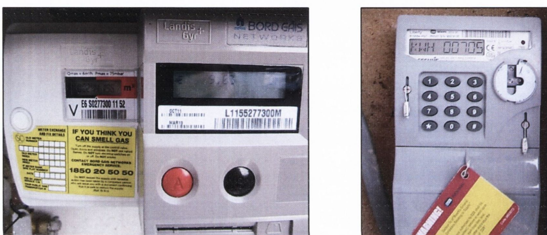
Figure 44 a) Landis+Gyr Libra 200 Series prepay meters b) Prepay electricity meter installed at Dwelling E
