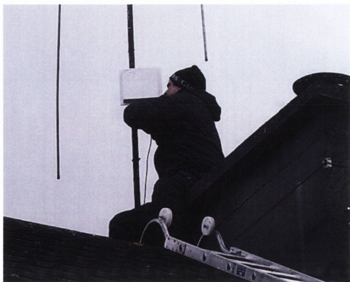
Figure 18 WAP connection located on the roof of each house to ensure visible line to antenna
