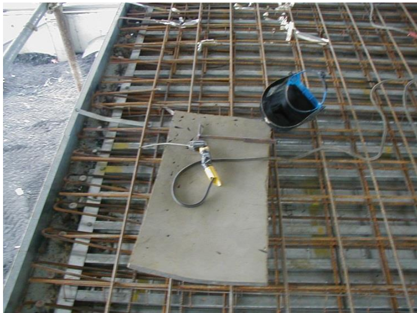
Fig 3.5.19.a. Photograph showing evidence of studs welded with sticks. The studs can be seen to the left of the photograph. (Confidential Source, 2015).
