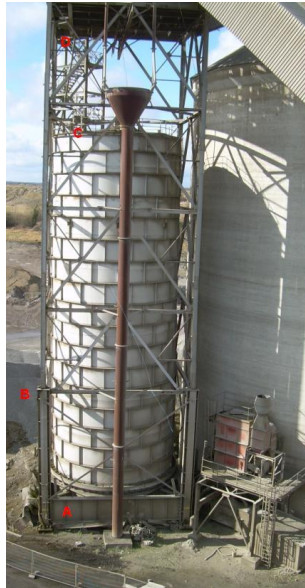
Fig 3.5.3.a. View of silo after failure (Confidential Source, 2015).
