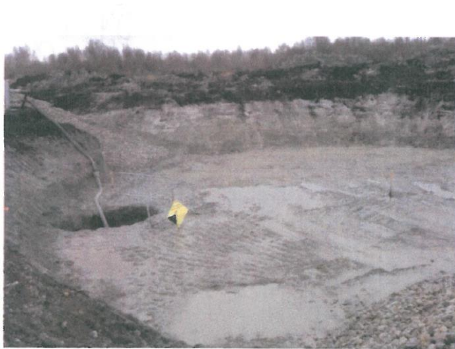
Fig 3.5.31.b. View of sinkhole – note water pump (Confidential Source, 2015).
