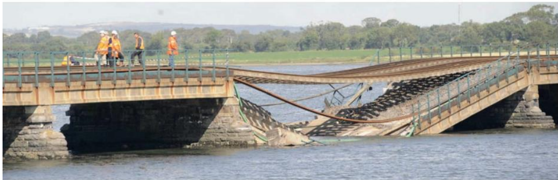
Fig 2.2.4.c The Viaduct after collapse (Institution of Structural Engineers 2012)
