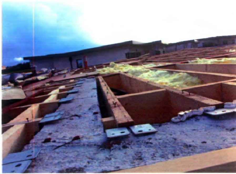
Fig 3.5.24.d. Additional view of damaged roof. (Confidential Source, 2015).
