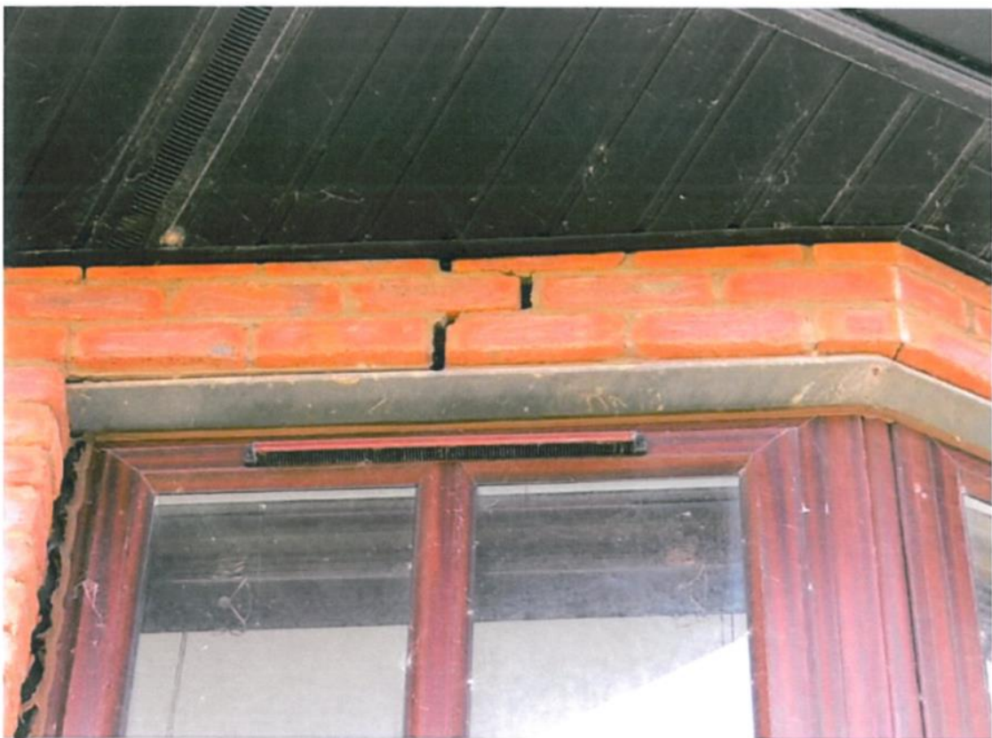
Fig 3.5.32.c. Front elevation – cracking over upper floor window. (Confidential Source, 2015).
