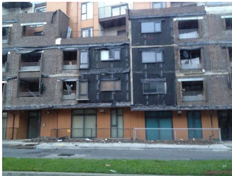
Fig 2.2.2.b Priory Hall (after investigation work) (TheJournal.ie, 2011)
