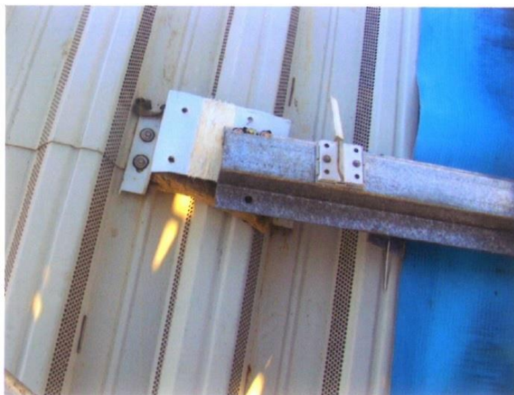
Fig 3.5.8.e. Damage to two top hat sections (Confidential Source, 2015).
