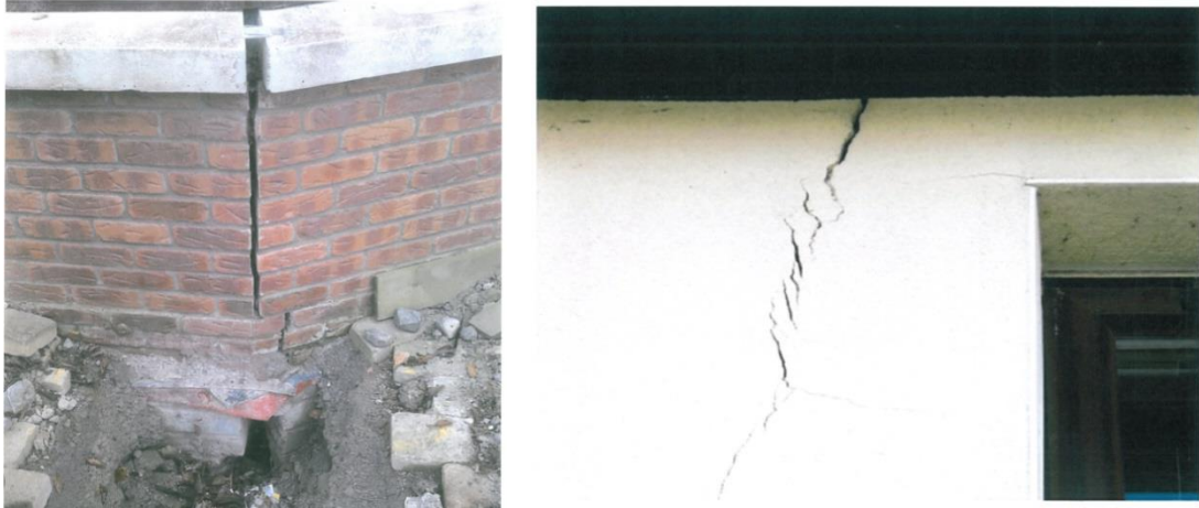
Fig 3.5.32.b. Cracks in front and rear elevations. (Confidential Source, 2015).
