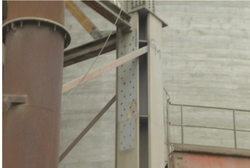
Fig 3.5.3.c. Failed bolted connection (Confidential Source, 2015).
