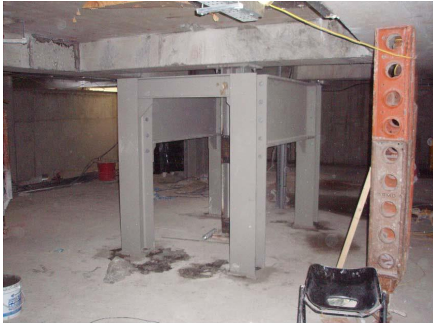
Fig 3.5.11.g. View at upper basement level showing emergency prop and temporary props (Confidential Source, 2015).
