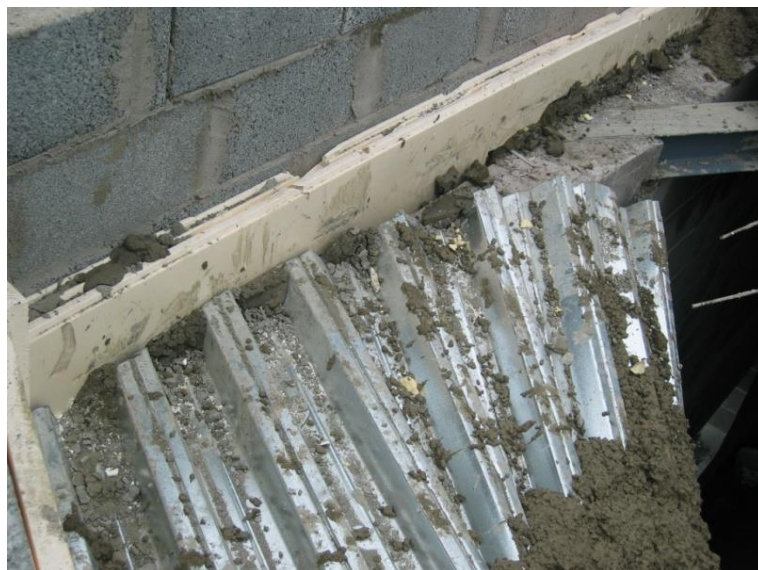
Fig 3.5.20.b. Photograph showing absence of cavity at external wall. (Confidential Source, 2015).
