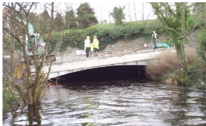
Fig 3.5.28.c. View after pile failure. (Confidential Source, 2015).
