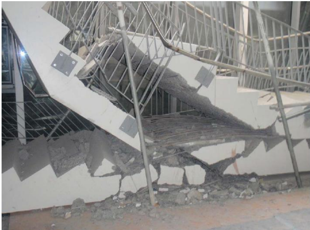
Fig 3.5.14.c. Collapsed stairs. (Confidential Source, 2015).
