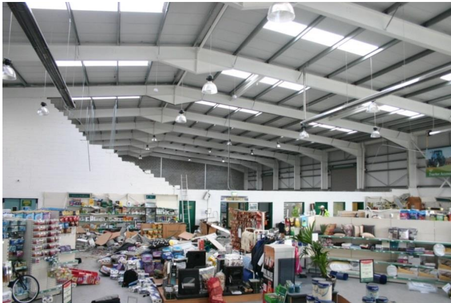
Fig 3.5.22.a. Internal view after the collapse. (Confidential Source, 2015).
