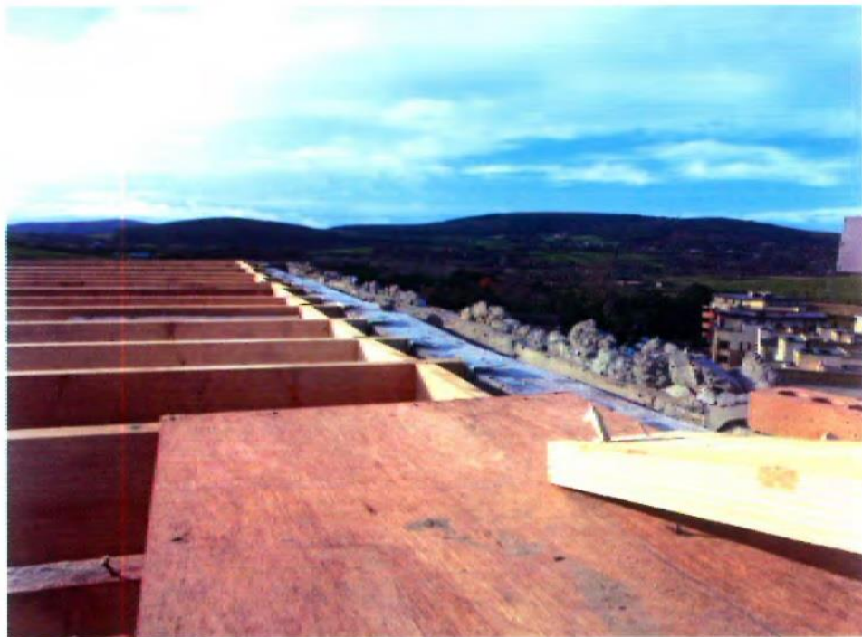
Fig 3.5.24.c. View of damaged roof. (Confidential Source, 2015).
