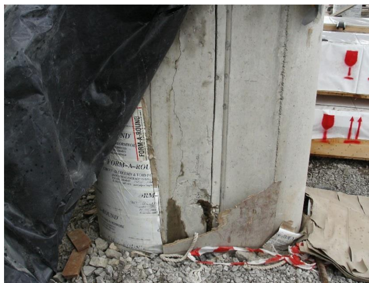
Fig 3.5.12.b. Photograph showing base of column and sawn cut. (Confidential Source, 2015).
