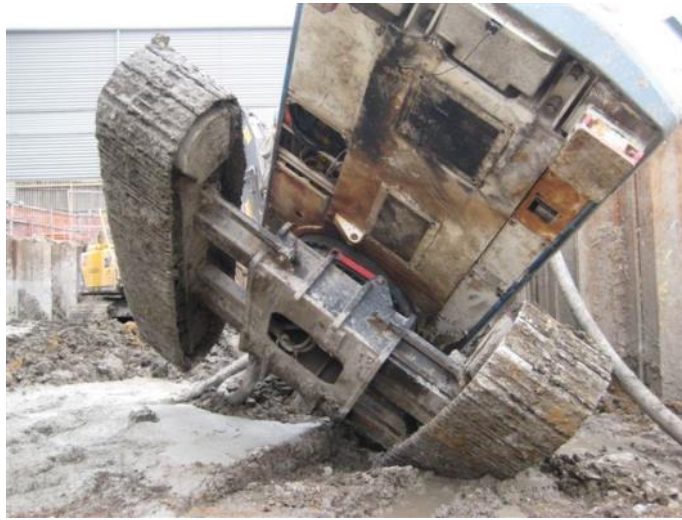
Fig 2.3.8.a Piling rig overturning (Construction Enquirer, 2015).
