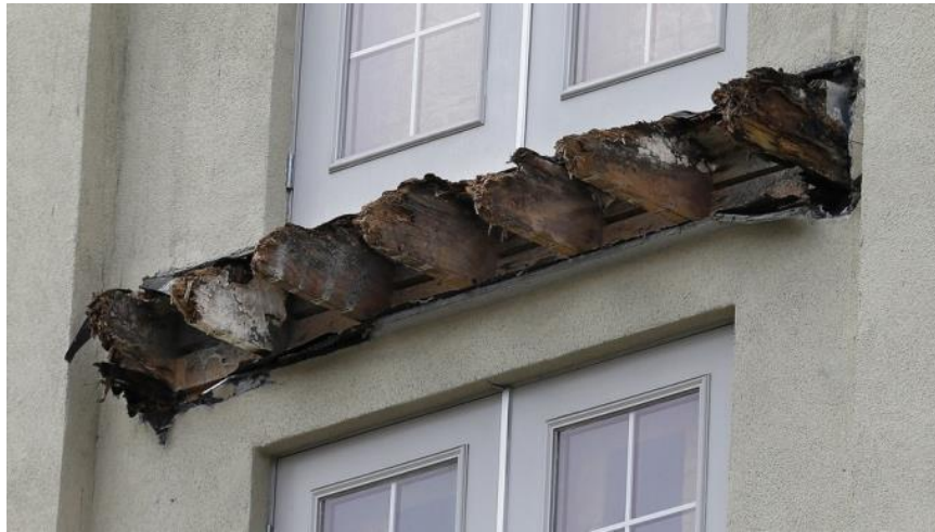
Fig 1.2.1 Fatal balcony collapse at Berkeley (TheJournal.ie, 2015)
