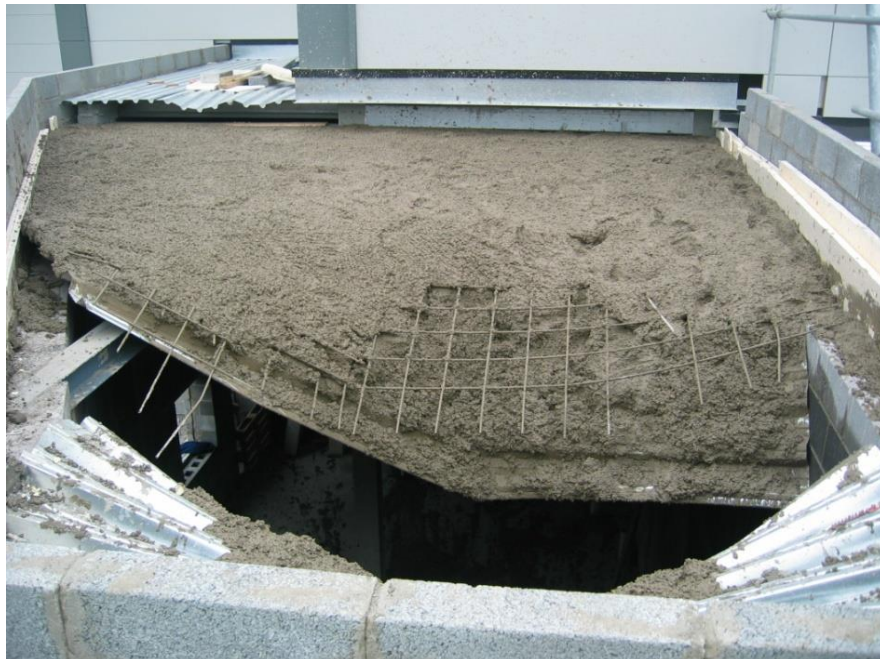
Fig 3.5.20.a. Deck failure during construction. (Confidential Source, 2015).
