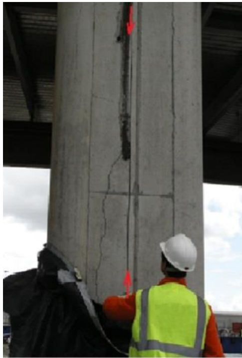
Fig 3.5.12.a. Photograph showing dislodged soft board and crack in concrete. (Confidential Source, 2015). (Sawn joint highlighted)
