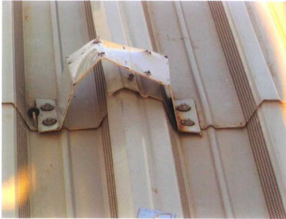
Fig 3.5.8.f. Damage to lower top hat section. (Confidential Source, 2015).
