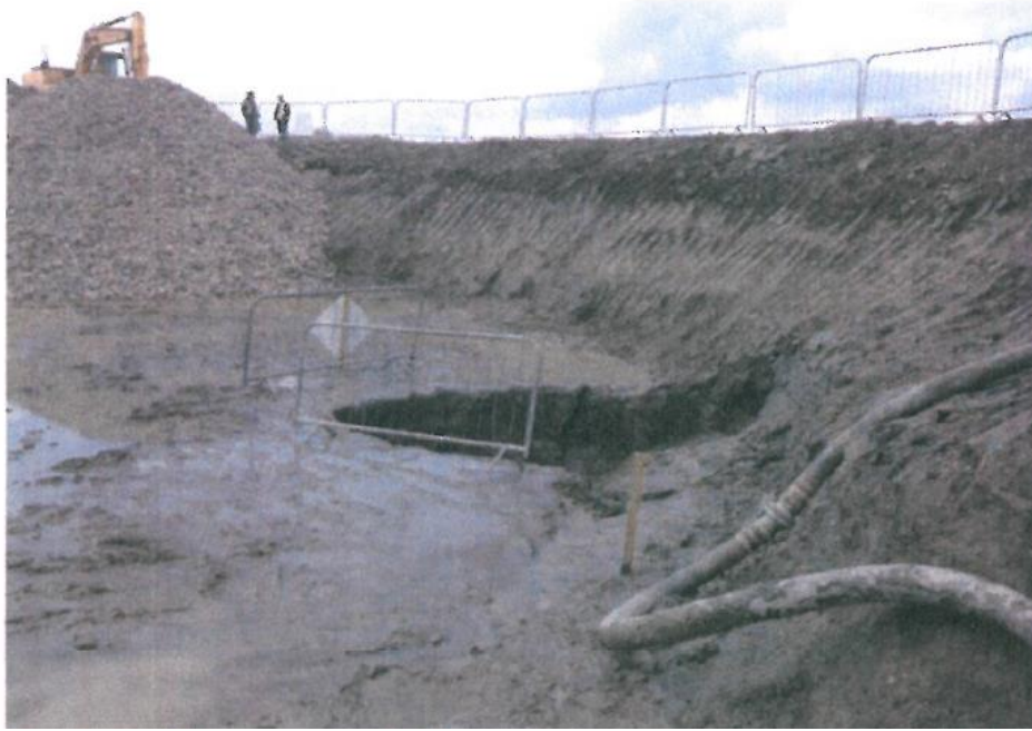
Fig 3.5.31.a. Photograph showing sinkhole during excavation work (Confidential Source, 2015).
