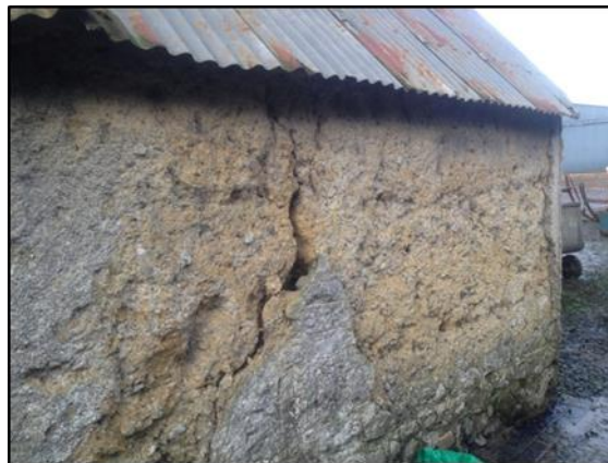
Figure 2: Staggered fractures across the wall.
