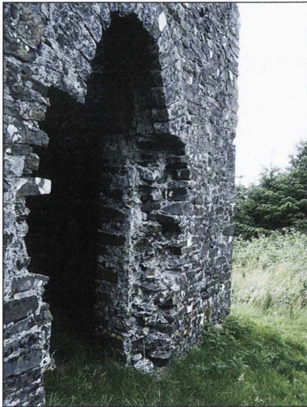
Figure 3.3.5: Results of Vandalism on Rear Archway
