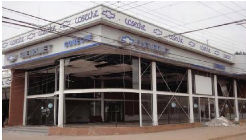
Figure 4-2 Damage windows and ceiling in a low-rise steel CBF in the Maule earthquake in Chile 2010 (Saatcioglu et al., 2013)
