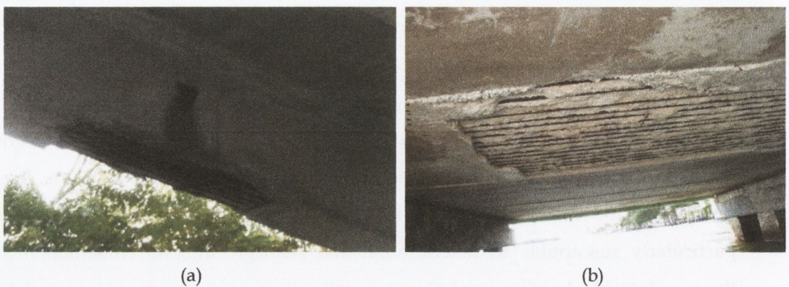
Figure 2.4 Corrosion of the underside of RC deck (Concrete Construction, 2011)
