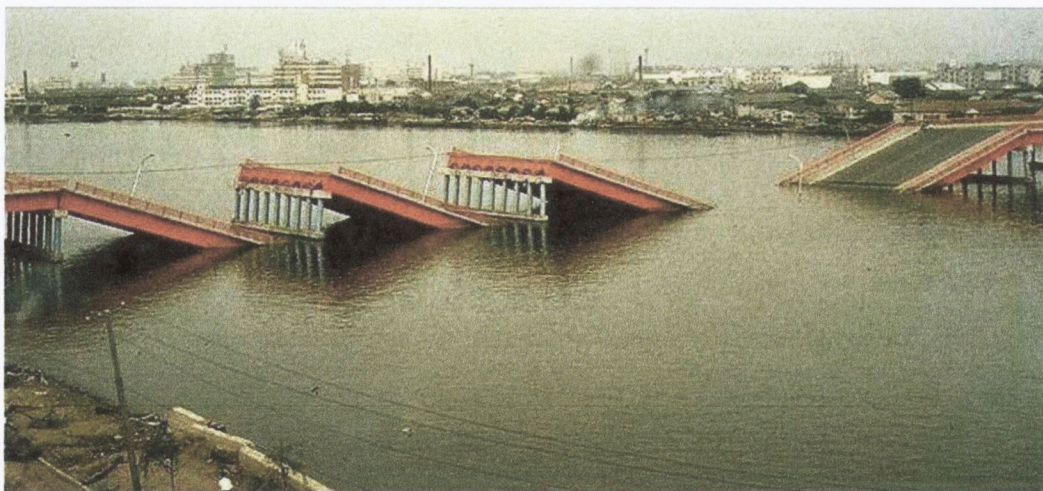
Figure 2.2 Deck unseating of the simply supported spans of the Showa bridge during the 1964 Niigata earthquake (Steinbrugge, 2011)
