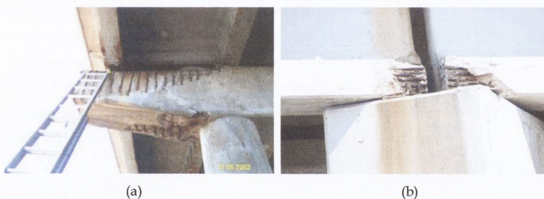
Figure 2.6 Corrosion of a bent cap and beam end due to the presence of joints (MTO, 2013, Howard Holland, 2012)
