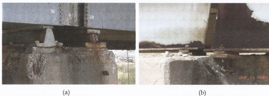
Figure 2.5 Corrosion of steel bearings (Freyssinet, 2013, Howard Holland, 2012)
