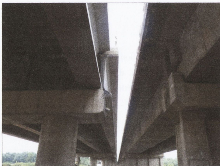
Figure 7.6 Damage to shear keys of two parallel bridges in the aftermath of the 2010 Chilean earthquake (Mosqueda, 2010)
