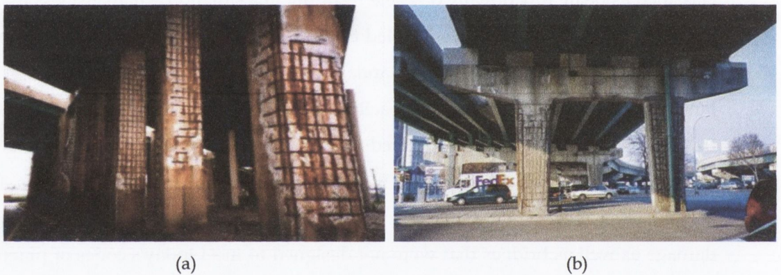
Figure 2.3 Corroding RC columns of highway bridges (Vector Corrosion Technologies, 2013, Aboutaha, 2012)
