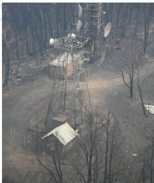
Figure 2: Burnt out communications tower – Mount Gordon Source: https://www.firelookoutsdownunder.com/Victoria/mtgordon.html
