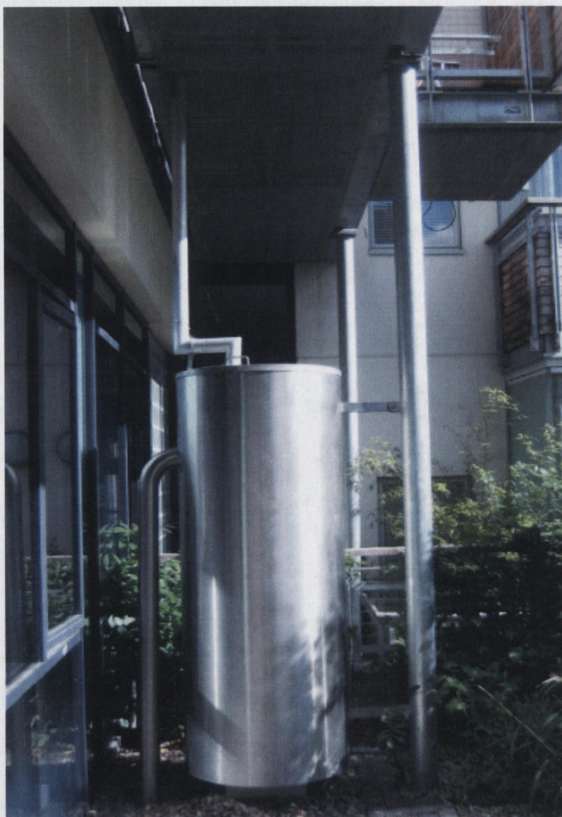
Figure18: Rain water harvesting tank York Street Dublin July 2010
