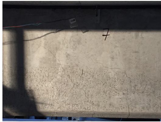
(b) PTB1-2 Close up of Cracking
