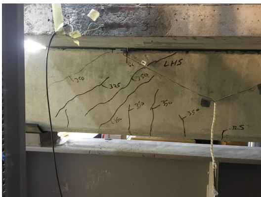
(c) PTB2-1 Cracks at 350 kN
