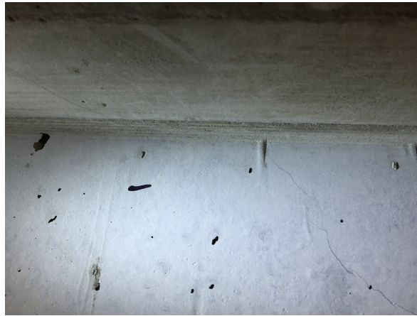
Figure 3.19: Close up of Interface Crack
