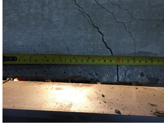
(b) PTB2-3 Cracking Measured
