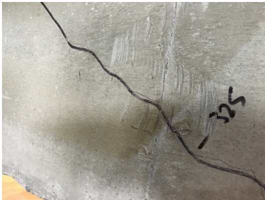
(a) PTB2-1 Close up of Crack
