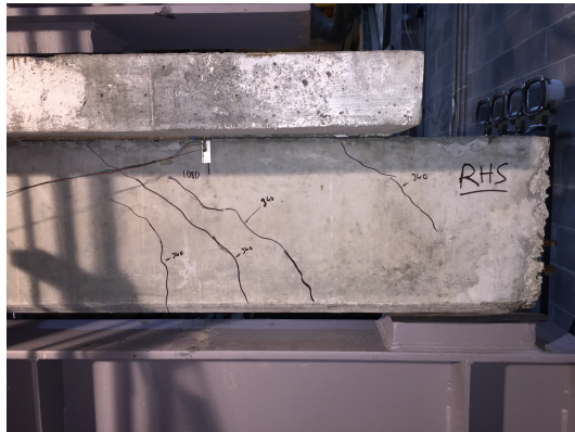
(a) PTB2-2 Cracking LHS
