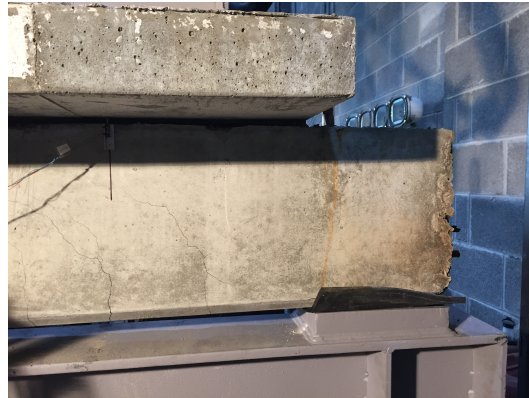
(b) PTB1-3 Cracking
