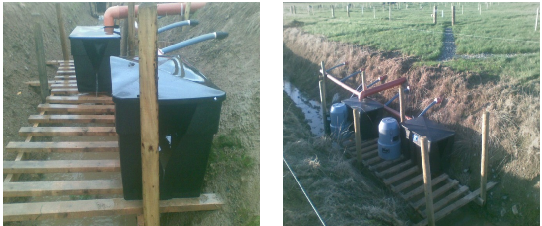
Figure X.8. Measurement tanks and flowmeters
