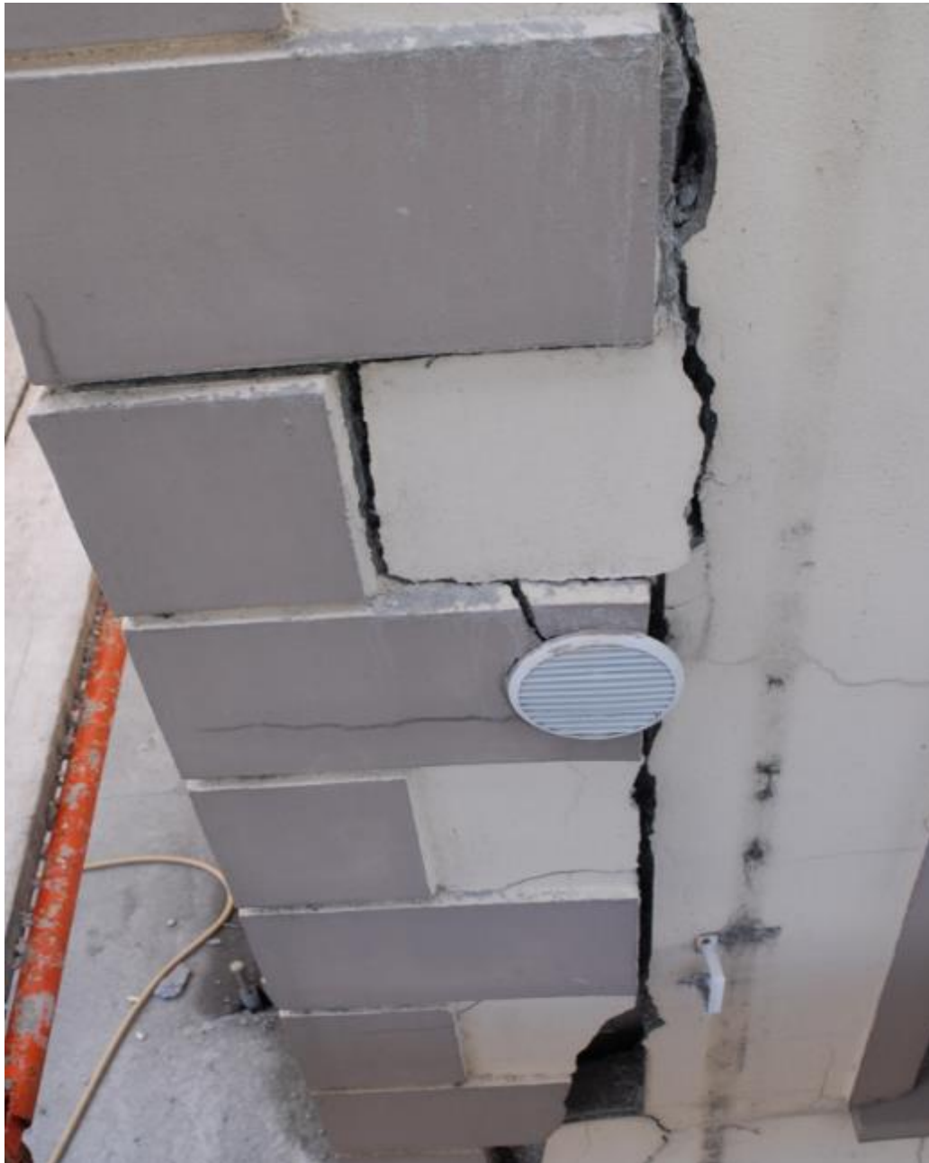
Figure 2: Severe vertical cracks in the gable end of a dwelling in County Donegal found to have high levels of mica in the concrete blocks used for its construction.
