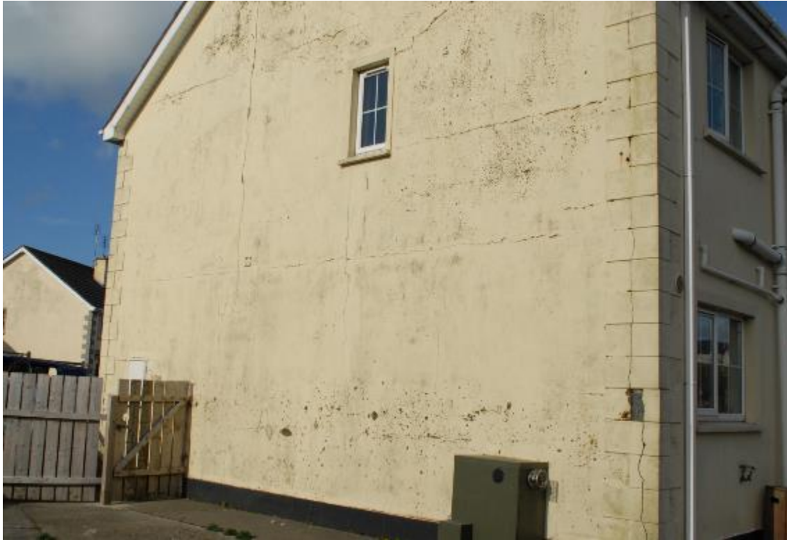
Figure 3: Gable end of a two storey semi-detached dwelling exhibiting the typical vertical and horizontal cracking pattern on the outer render, and a significant vertical crack through the quoin.
