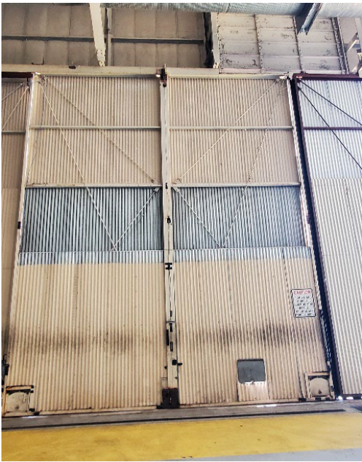
Figure 1: Rolling-hangar door used in this study.
