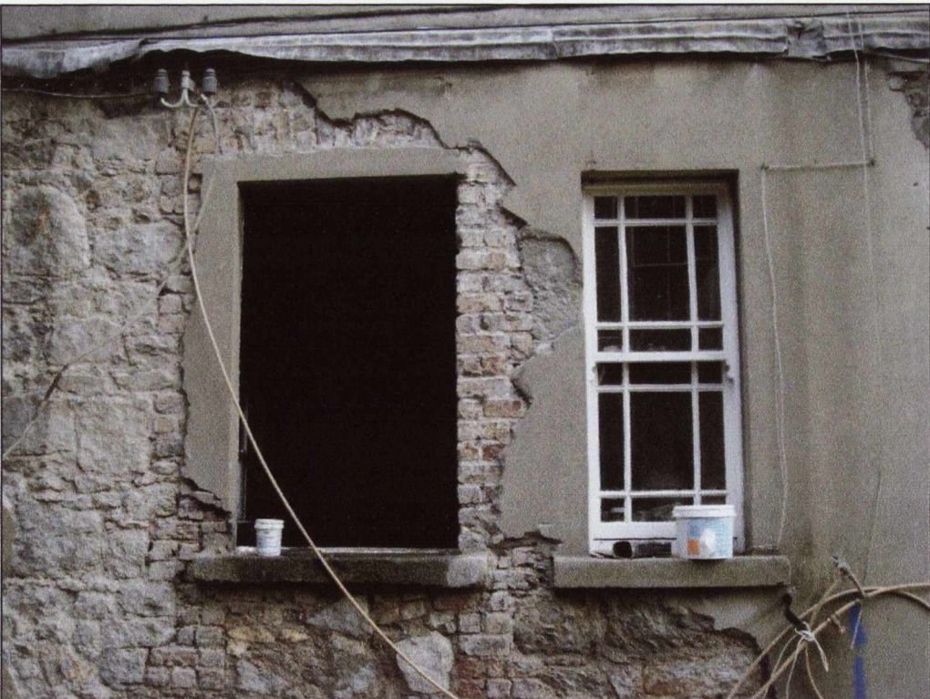
4.12: Number 7 Ailesbury Road: lower level, showing where openings in the granite wall were formed in brickwork.
