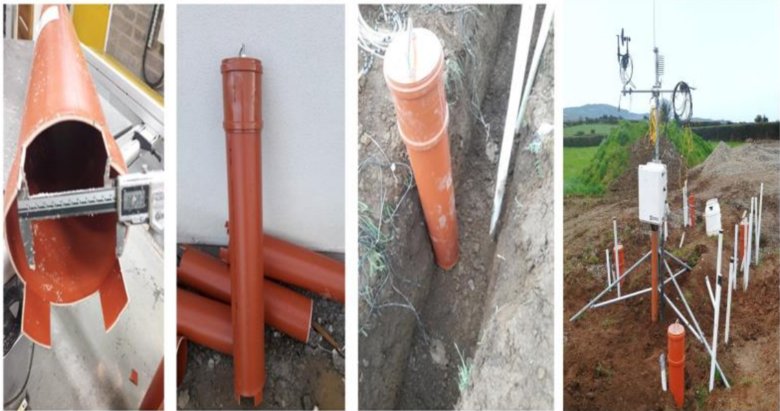
Figure 3.28. Construction of bioports with 100 mm wide inlets to permit effluent transport into the bioports area (left) profile of the bioports including port access lid (centre-left) installation of the port within the STU percolation trench (centre right), positioning of 1 m and 5 m bioports for trenches 2 and 3 within the Site C post construction.
