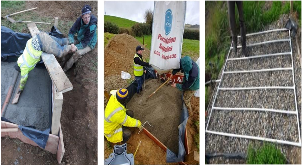
Figure 3.11 Construction of the open intermittent sand filter at Site C from its basic frame and sloped base and collection pipe to the STU (left), controlled addition of the percolation sand (centre), addition of percolation pipe manifold over gravel surface (right).
