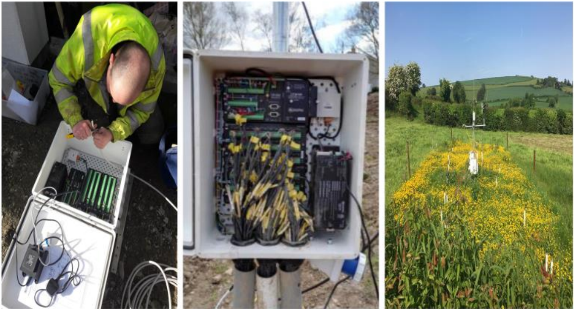
Figure 3.13. Weather station during site build with multiplexer configuration barometer and power supply (left) soil moisture cables attached to multiplexers, backup battery supply and barometer (centre), complete installation on-site (right).
