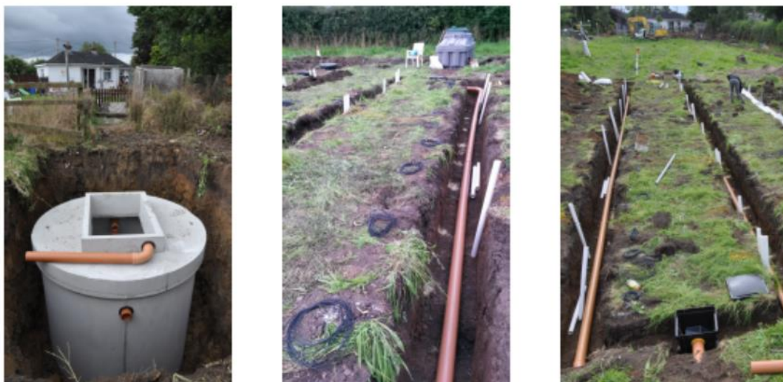
Figure 3.2. Construction of the on-site system in Site A, with the installation of the septic tank (left) , coconut husk filter (centre) and the distribution buckets and STU trenches (right)
