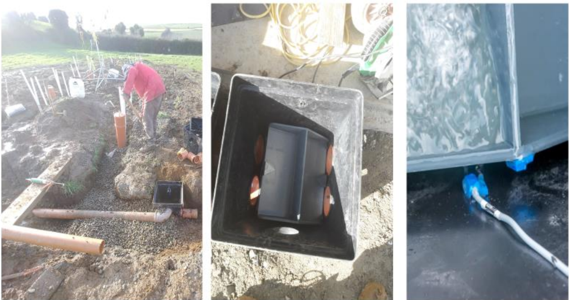
Figure 3.14. Installation of distribution boxes during site C build inlet effluent pipe is visible and leading towards one of the boxes (left) distribution box prior to installation with tipping bucket present (centre) blue reed switch magnets and communication cable installed to tipping bucket and distribution box (right).
