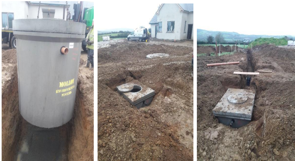
Figure 3.11. Installation of septic tanks (left), sand filter sump relative the septic tank and household (centre) and STU percolation trenches relative to the sump position (right).
