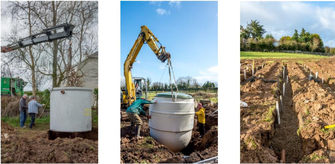
Figure 3.6. Installation of septic tanks (left), RBC (centre) and STU percolation trenches (right)
