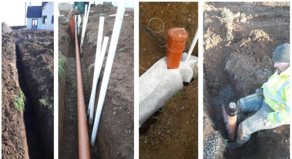
Figure 3.12. Construction of STU trenches at Site C (left) placement of percolation pipe (centre-left), application of geotextile membrane (centre right) and backfill with pea gravel and topsoil (right).
