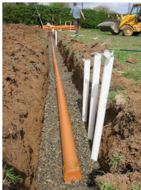
Fig. 2. Construction of percolation trench. Note white guide tubes for installation of lysimeters.
