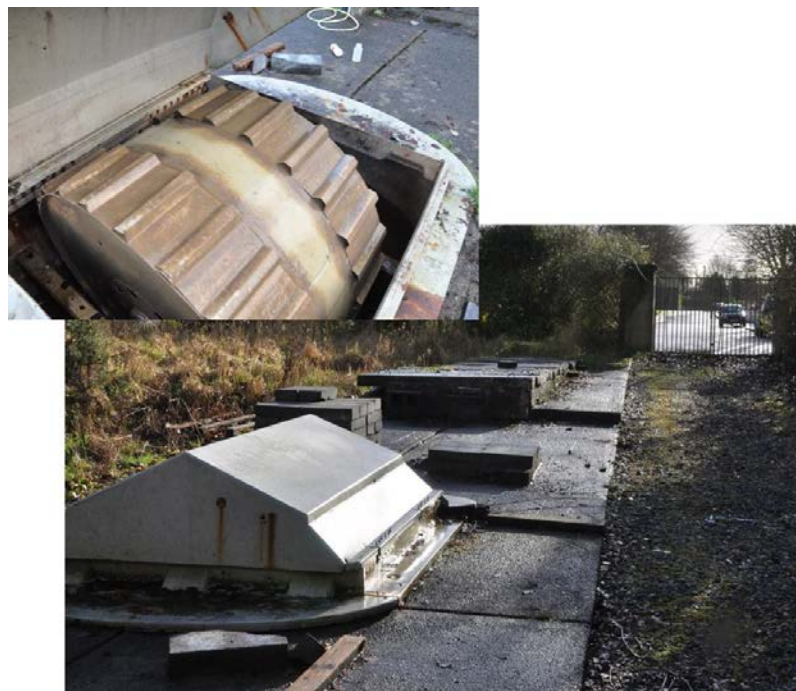
Figure 3.26 Treatment Plant with view of rotating media disc (insert) at Toonagh, Co. Clare
