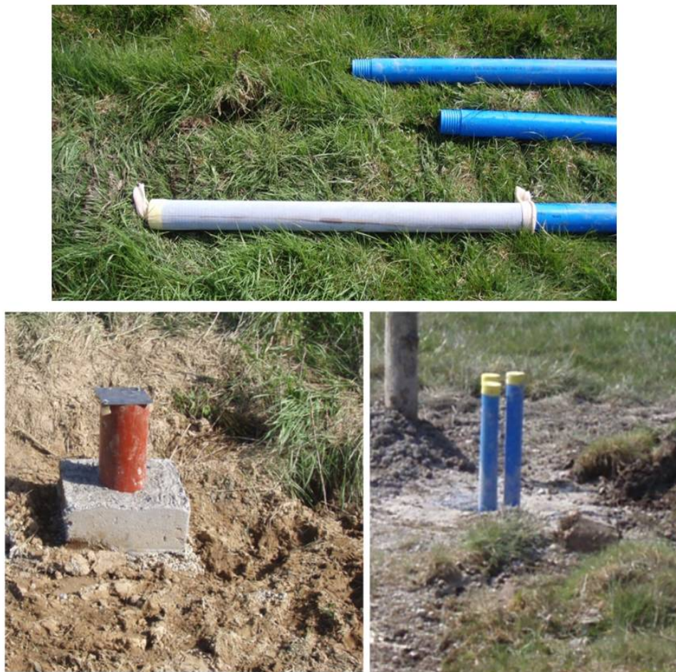
Figure 4.10 (a) Piezometers prior to installation with geo-membrane covering slotted section (b) Completed Borehole with raised cover and concrete plinth (c) Installed piezometers during borehole construction
