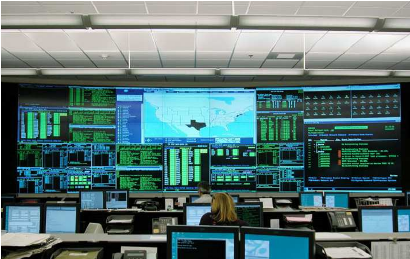
Figure 5.4: An example of a dedicated control facility for system operations
